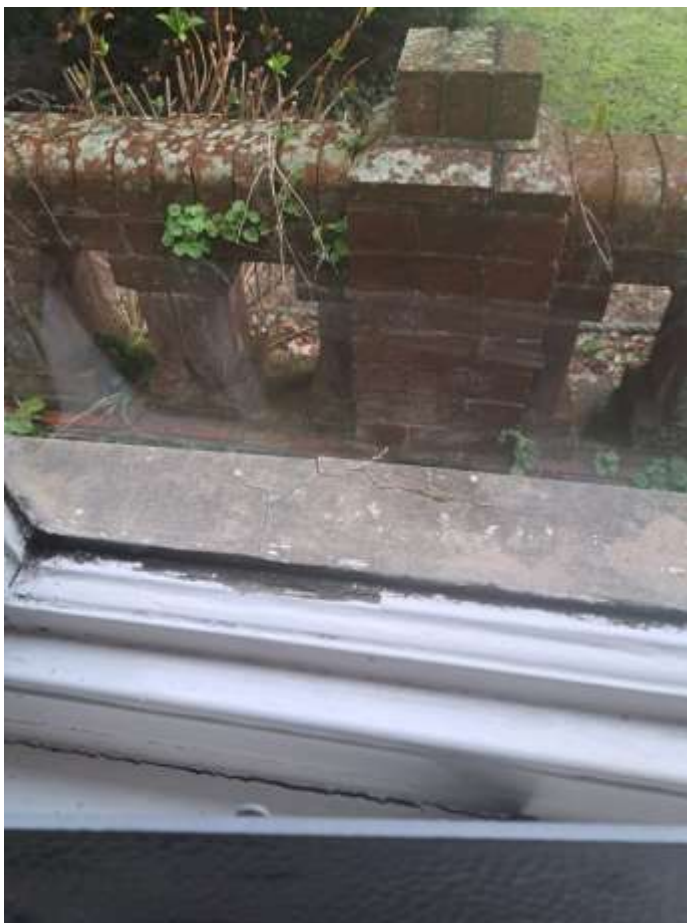
Photo 9 - more rotten windows
