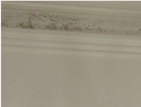
Photo 13 - More ceiling mould
