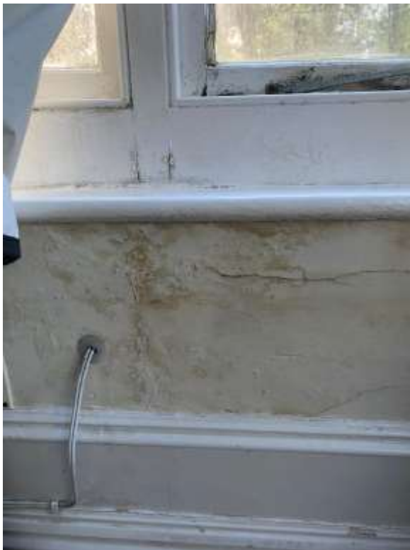
Photo 7 - Another downstairs flat. Drain pipes flooded due to lack of guttering cleaning and care.
